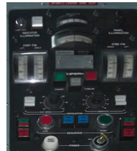
Non-supported Bridge Analog Control Panel
